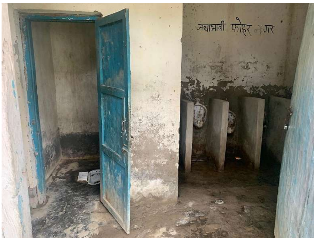
Situation of toilets in one of the public schools of Durgabhagwati Rural Municipality, Rautahat
